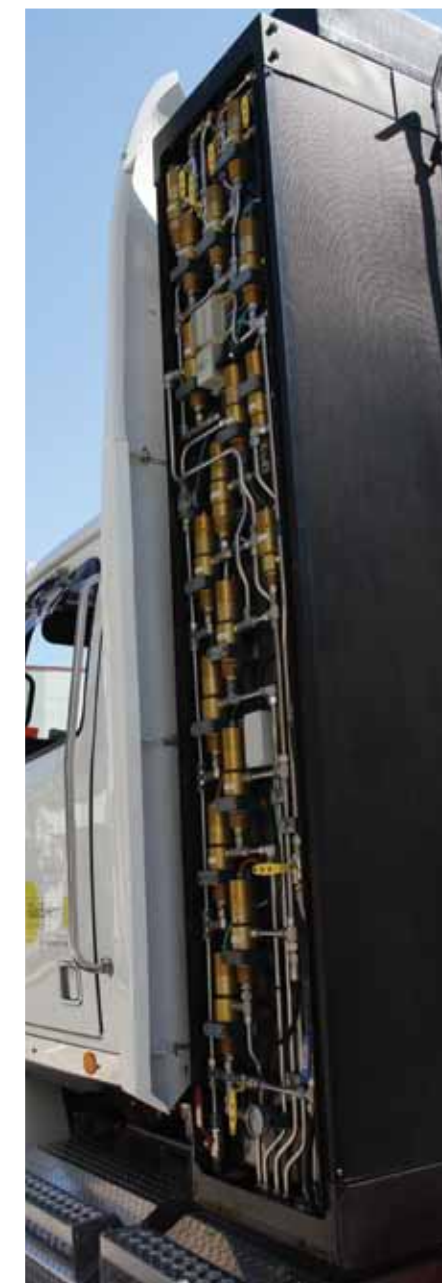
The myriad of pipes, valves and dials that hides under the side cover of the fuel pack
